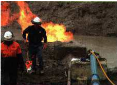
Gas from the Walloon Coal Measures will fuel a new power station at Blackwater.
